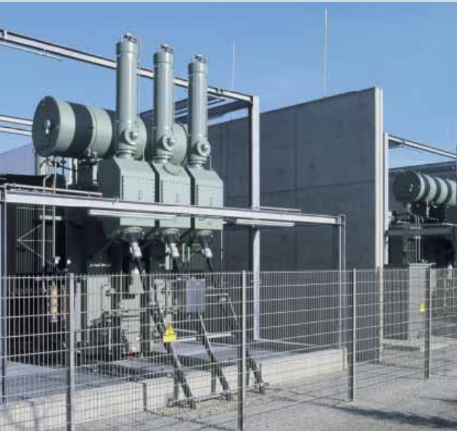
GIS arresters installed at a 123 kV transformer with Oil-SF 6 -bushing
