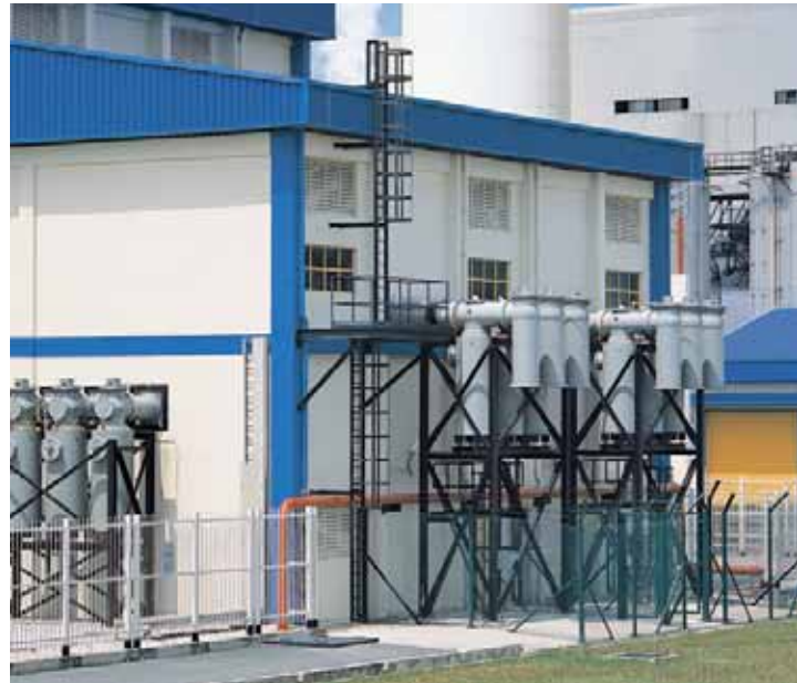
GIS arresters connected to a 420 kV GIS busbar
