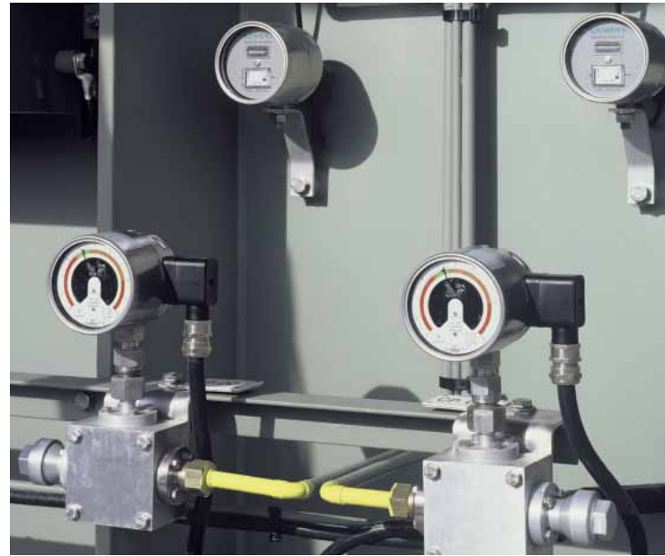
Gas and electrical monitoring for GIS arrester
